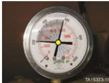
Figure 32. Pressure gauge with pump speed too fast wide swing in pressure (cavitation occurs)
