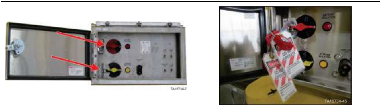
Figure 47. Battery Isolation Box – Battery isolation switch in OFF position with locks in place
