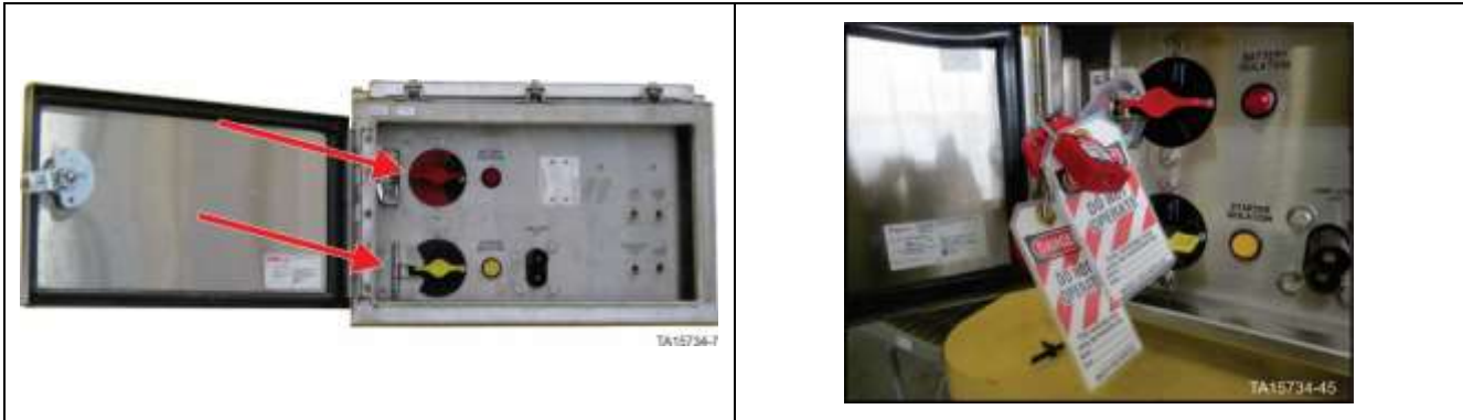
Figure 70. Battery Isolation Box – Battery isolation switch in OFF position with locks in place
