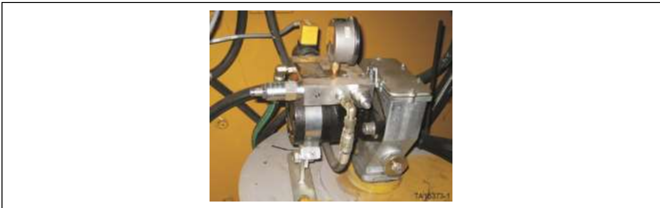
Figure 3. Typical auto lube grease pump
